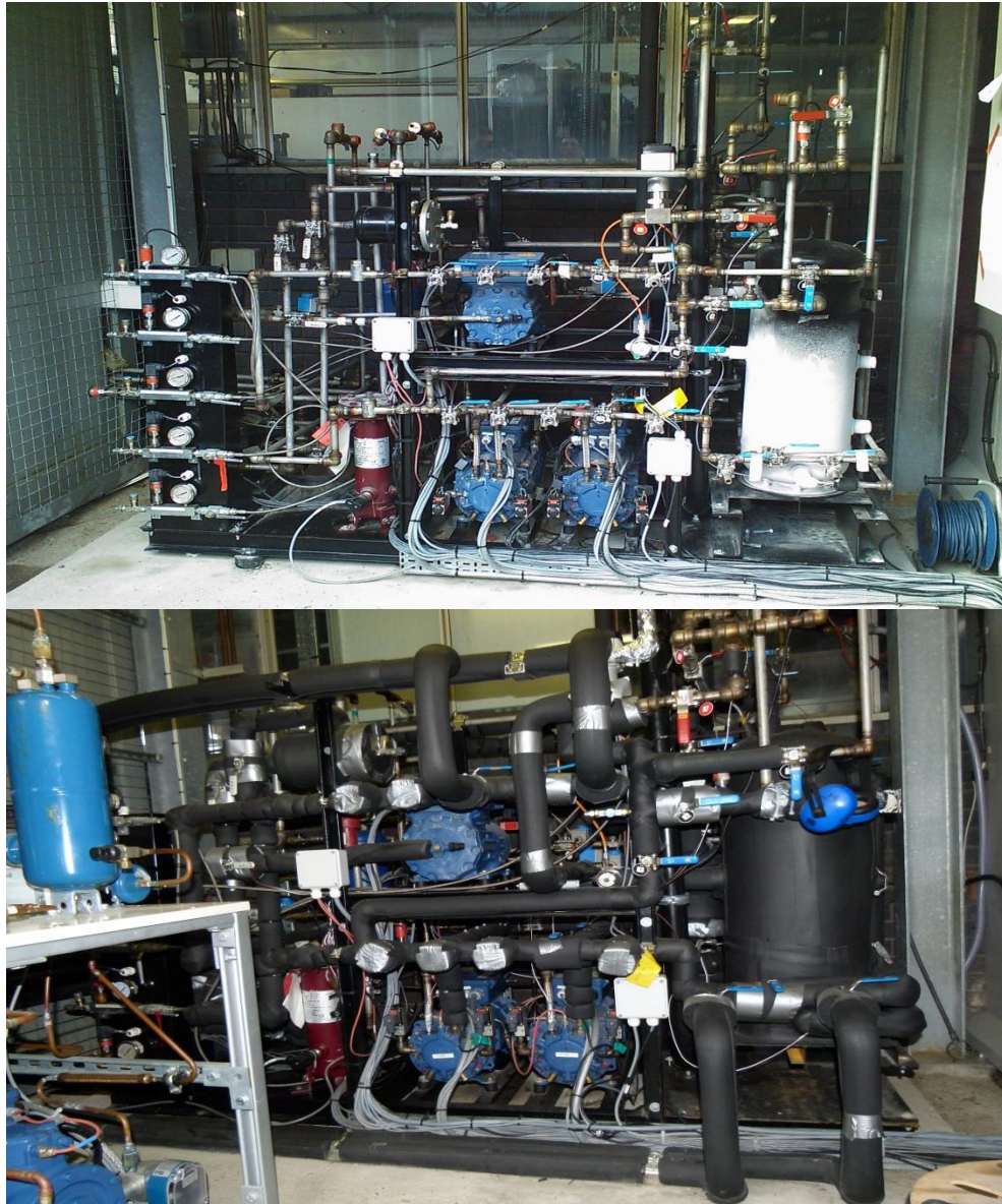
Figure 5.2 CO 2 booster experimental test rig
