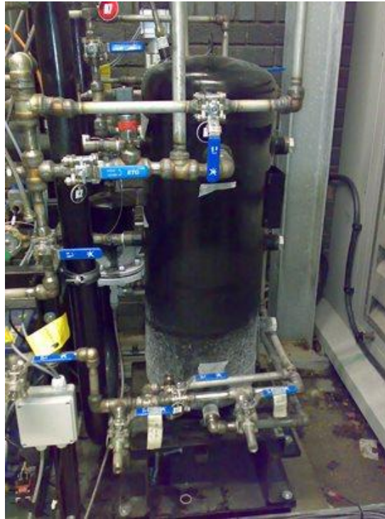
Figure 5.17 Liquid receiver installed in CO 2 system
